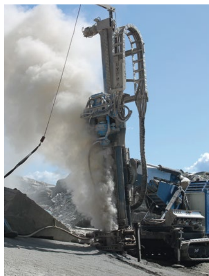
VD100 drilling in medium-hard rock, 100 m deep, hole diameter 135 mm, flushing with air
