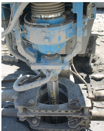
VD100 drilling in granite, 25 m deep, hole diameter 120 mm, flushing with air
