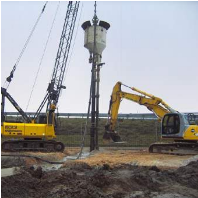
Crane suspended application for dry bottom feed stone columns in Chioggia Italy.
