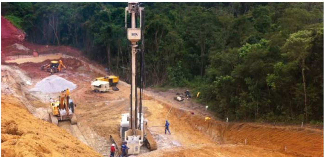
Piling rig application for dry bottom feed stone columns in Sao Paulo Brasil.
