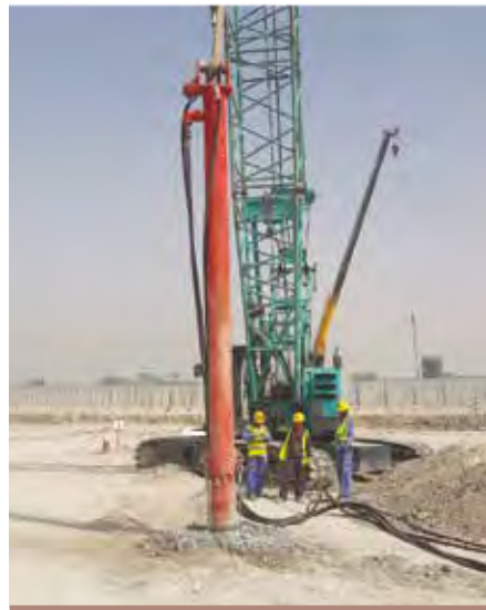
900 stone columns realized with a VL18 Vibrolance for the foundation of a new school in Sharjah, UAE. Those column was installed with a triangular grid of 2.5m, 4m deep within 3 weeks.
