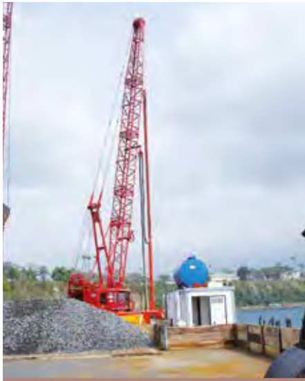
Two Vibrolances doing top feed stone columns under water at 17 m depth for the Malabo Harbor, Equatorial Guinea .
