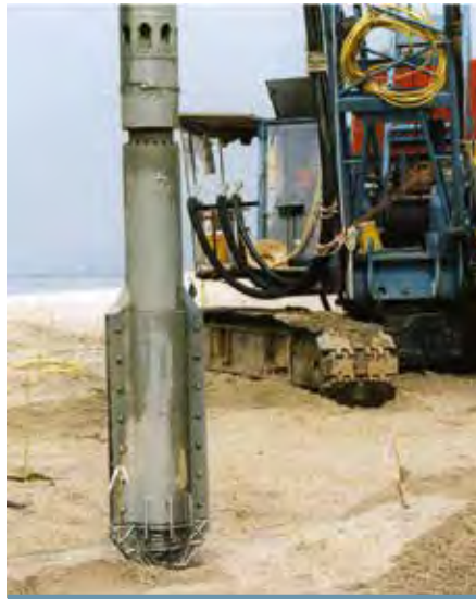
Vibrolance VL110 working at 31 m depth to compact 2,000,000 m 3 of land reclamation for the extension of the LAMME power station, Hong Kong .
