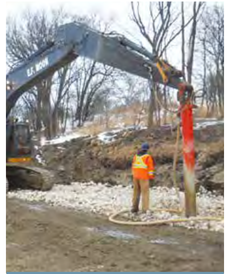
VL18 Vibrolance in a deep compaction works of a 7 m depth for a river bank stabilization in Canada .
